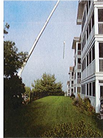
An enormous crane raises materials to the roof as part of the replacement project of HVAC units for the South, Central and North Wings.
